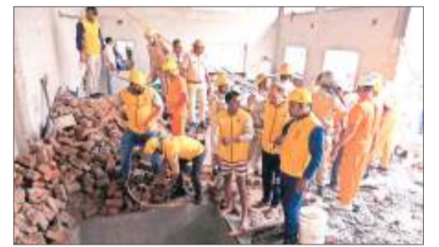
Rescue work underway after a wall of an under-construction house collapsed, in Subhash chowk area of Jaipur, Monday. ROHIT JAIN PARAS
