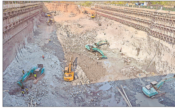
A major component of the project is the 5.3-km-long twin tunnels to be constructed beneath the Sanjay Gandhi National Park. EXPRESS
